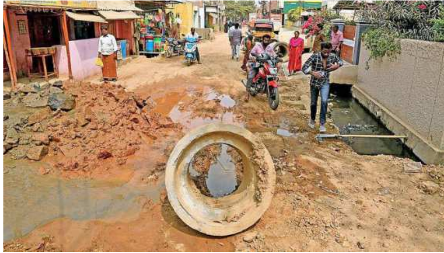
The Line Road between Linemedu and Shevapet Police Station in Salem has become a commuters' nightmare due to the long drawn-out underground drainage works. E LAKSHMI NARAYANAN
